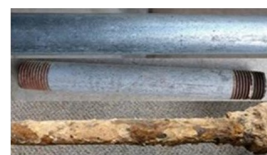
Galvanized pipes are dull gray and a strong magnet will stick to the pipe
