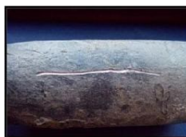
Lead pipes are dull gray and very soft and look like a new nickel when scratched or
